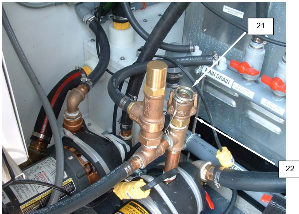
Figure 16. P-1 Pump Priming Standpipe.
