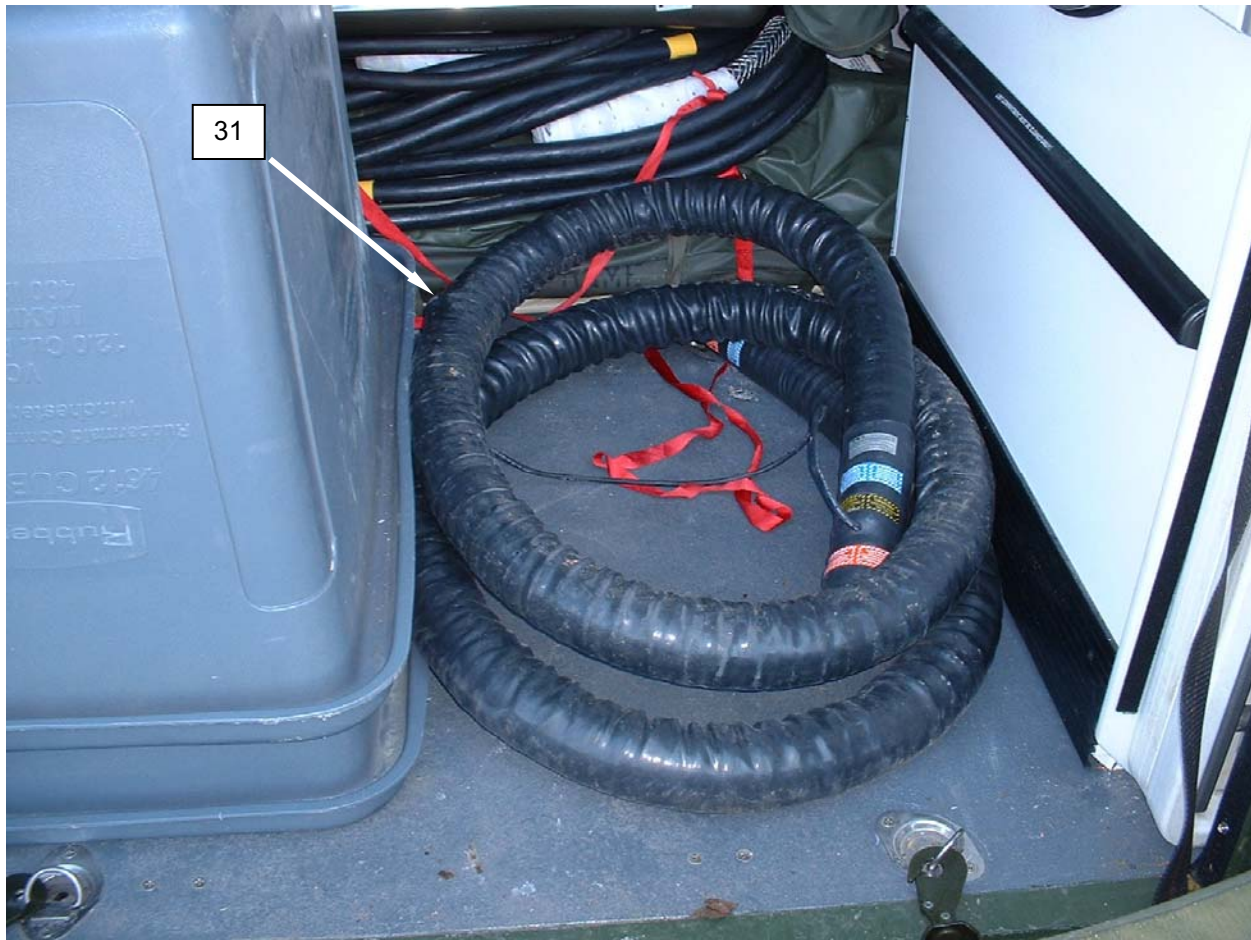
Figure 27. Heat Trace Hose on Floor.
