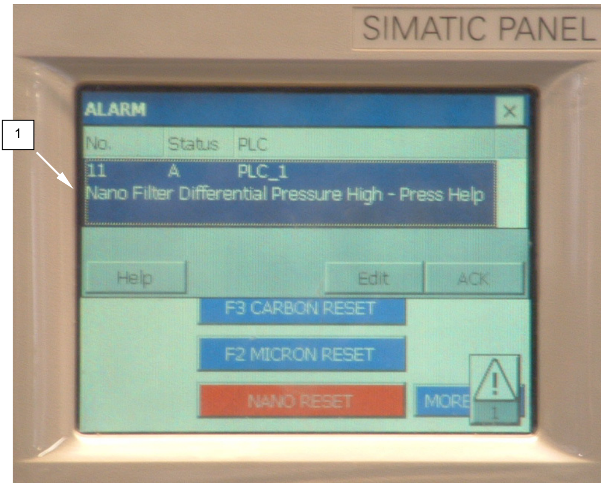
Figure 20. Nano Filter Differential Pressure High Alarm on PLC Display.
