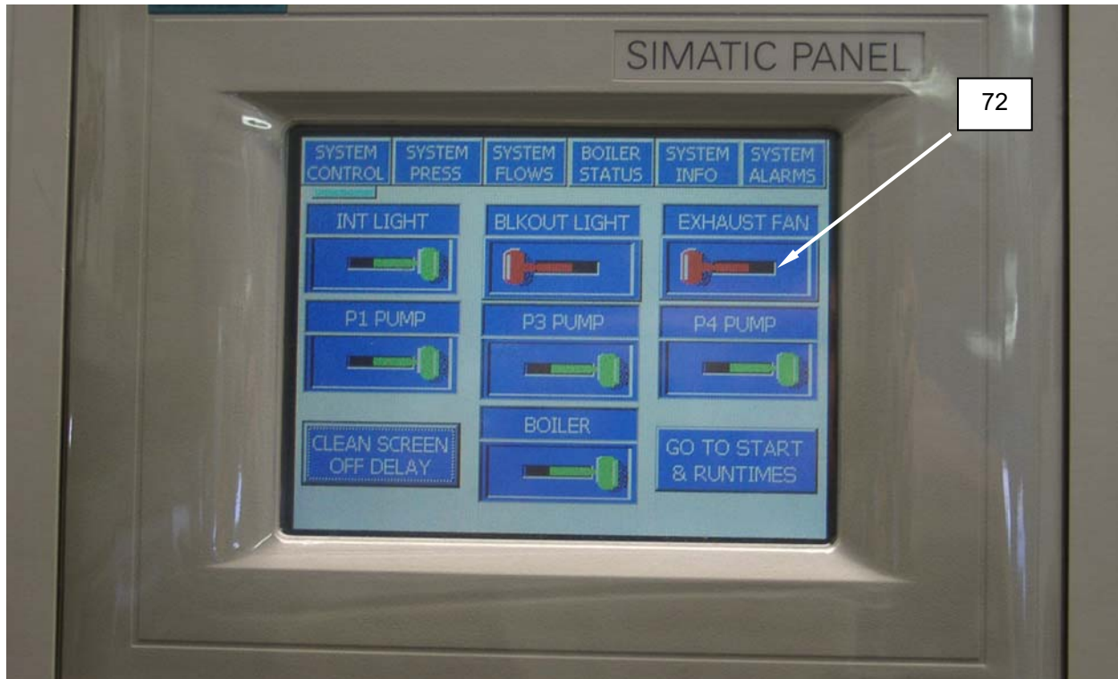
Figure 29. Operate the Exhaust Fans.
