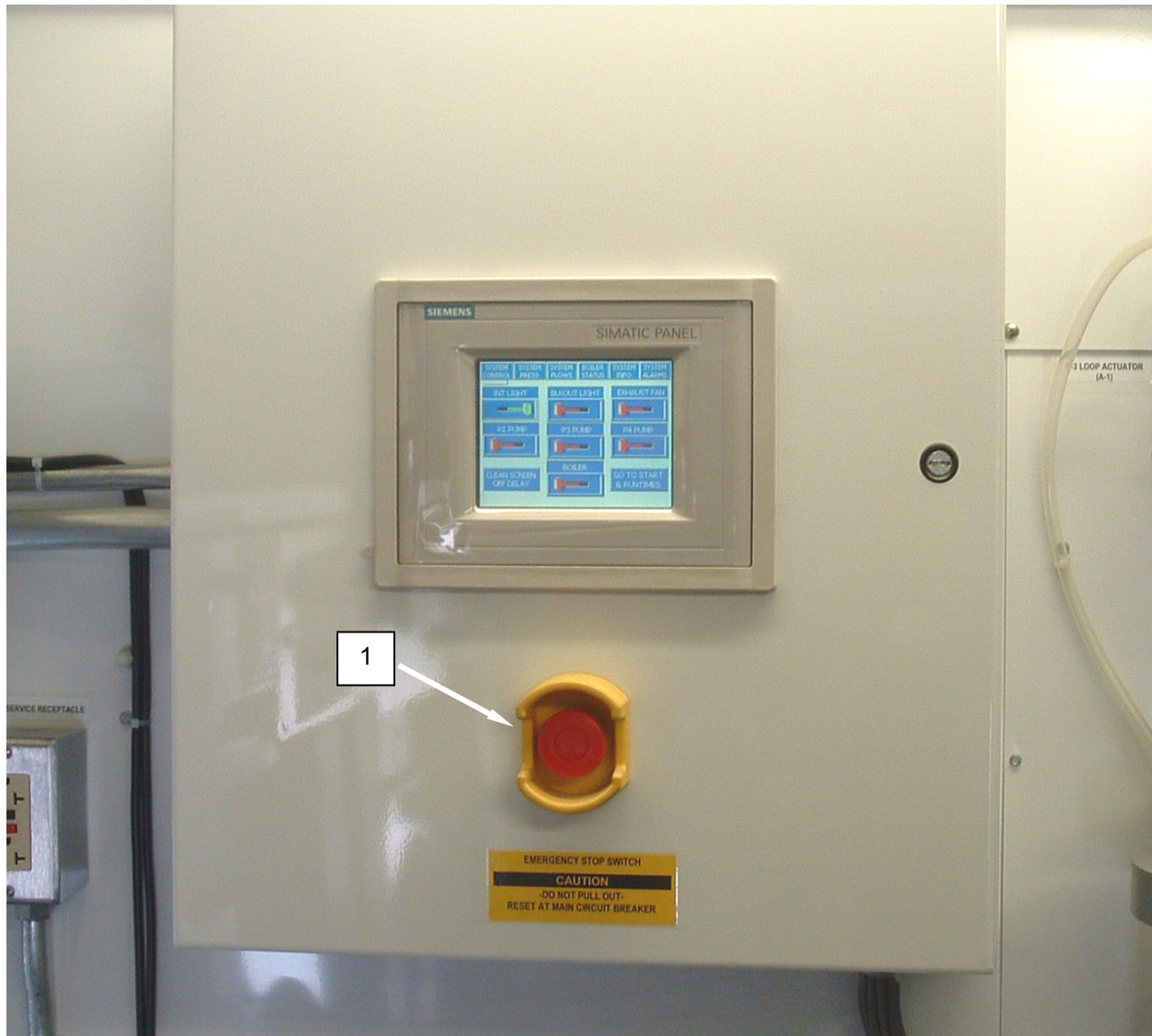
Figure 1. Emergency Shutdown Switch.
