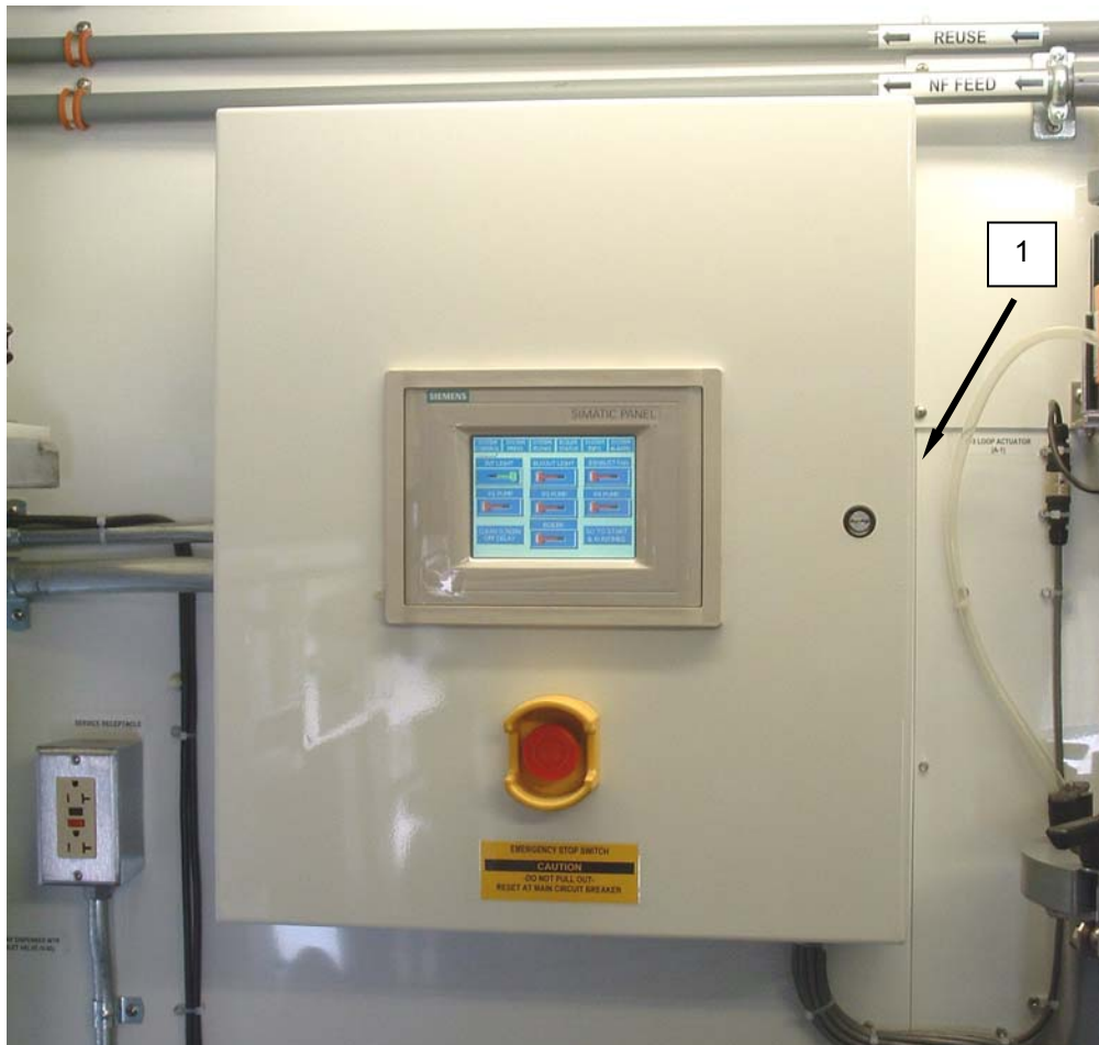
Figure 1. PLC Control Panel.
