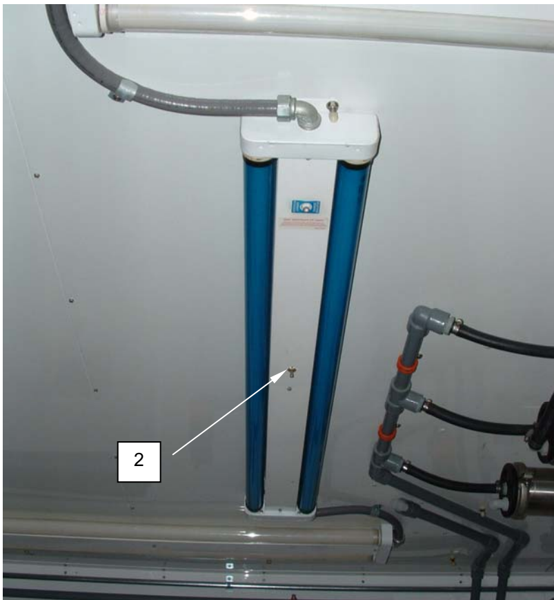
Figure 2. Switch on the Battery Backup for Emergency Lighting.
