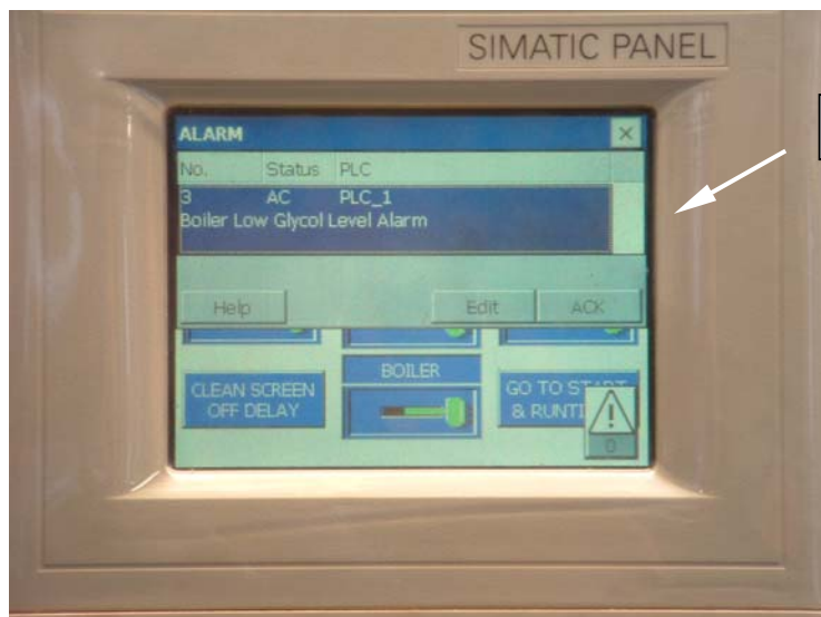
Figure 31. Boiler Low Glycol Alarm on PLC Display.
