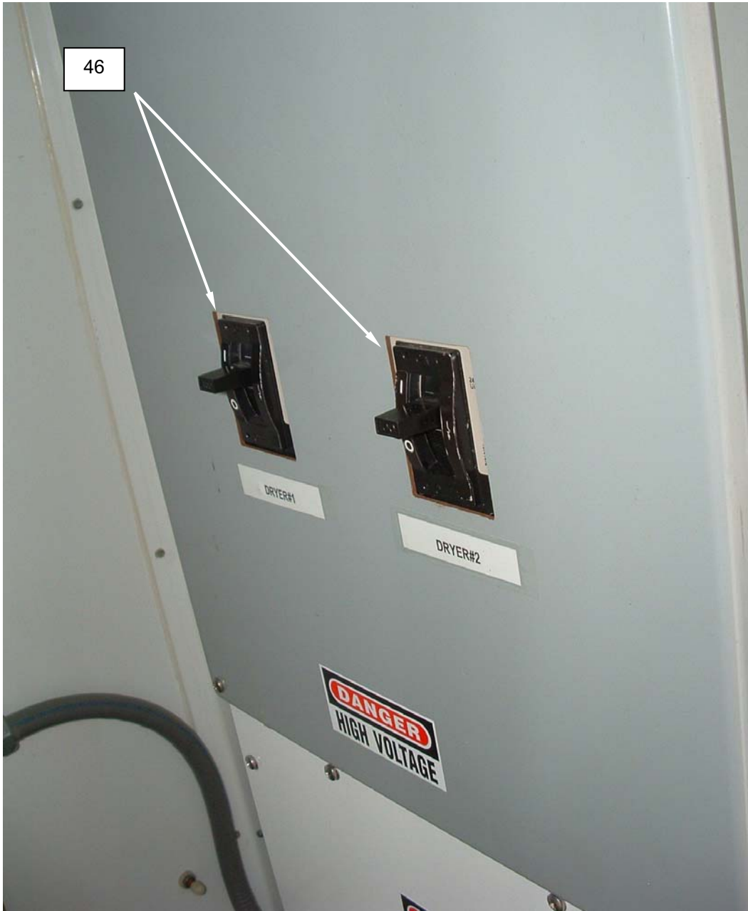
Figure 16. Dryer Circuit Breaker Panel.
