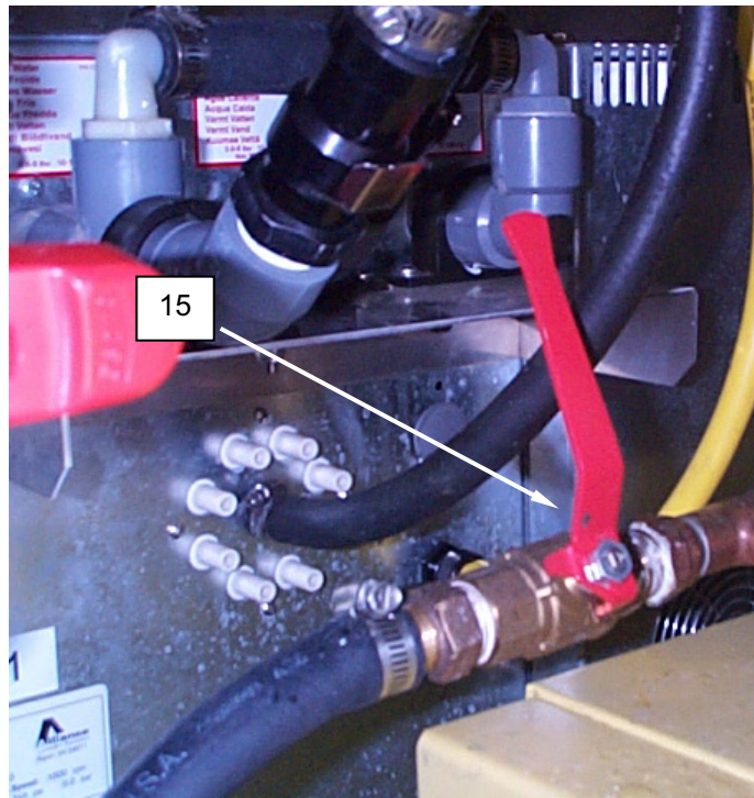
Figure 9. Boiler Water Outlet Drain Valve.
