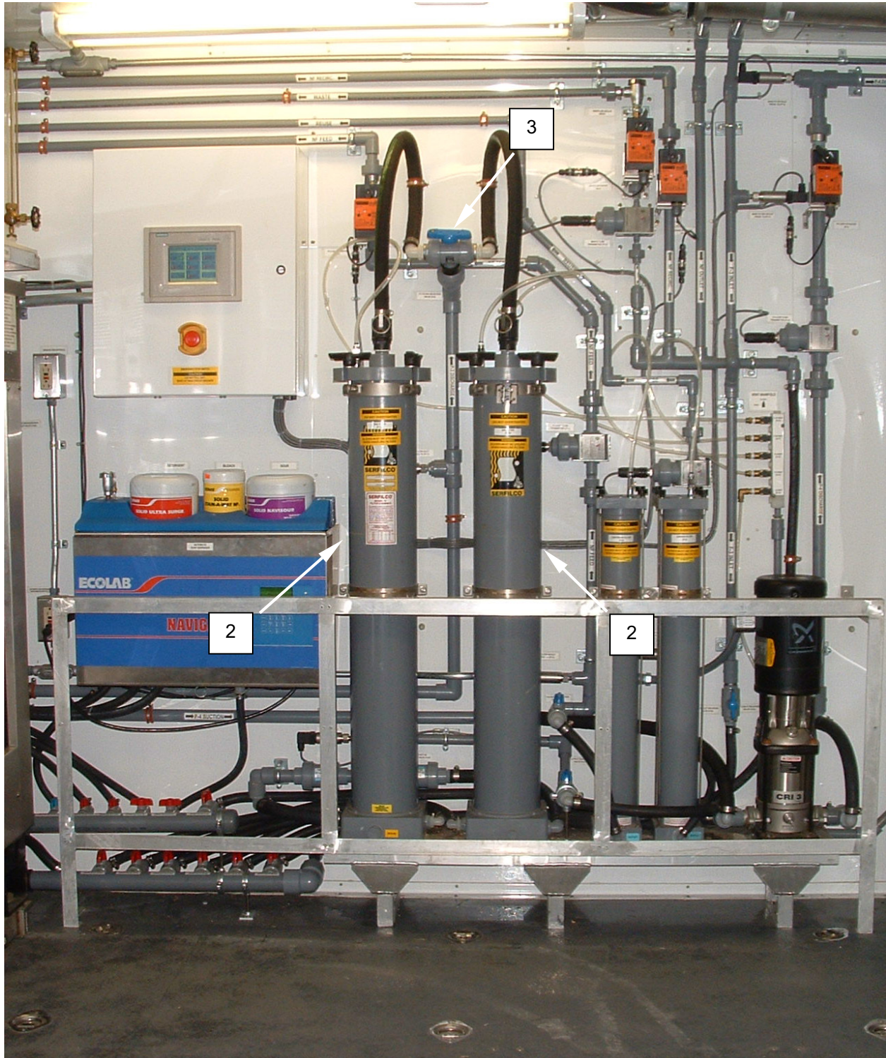
Figure 5. F1 Bag Differential Pressure High on PLC Display.
