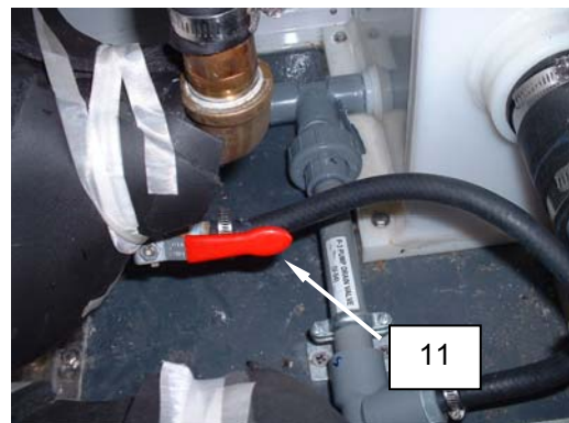
Figure 8. P-3 Pump Drain Valve.
