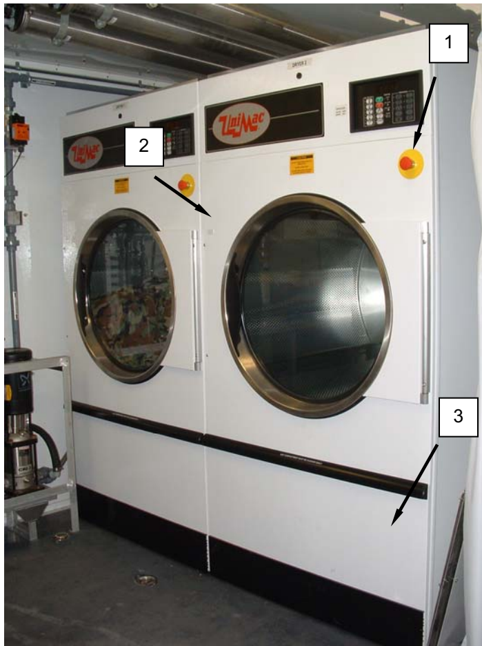
Figure 2. Dryer Drum doesn't Turn.
