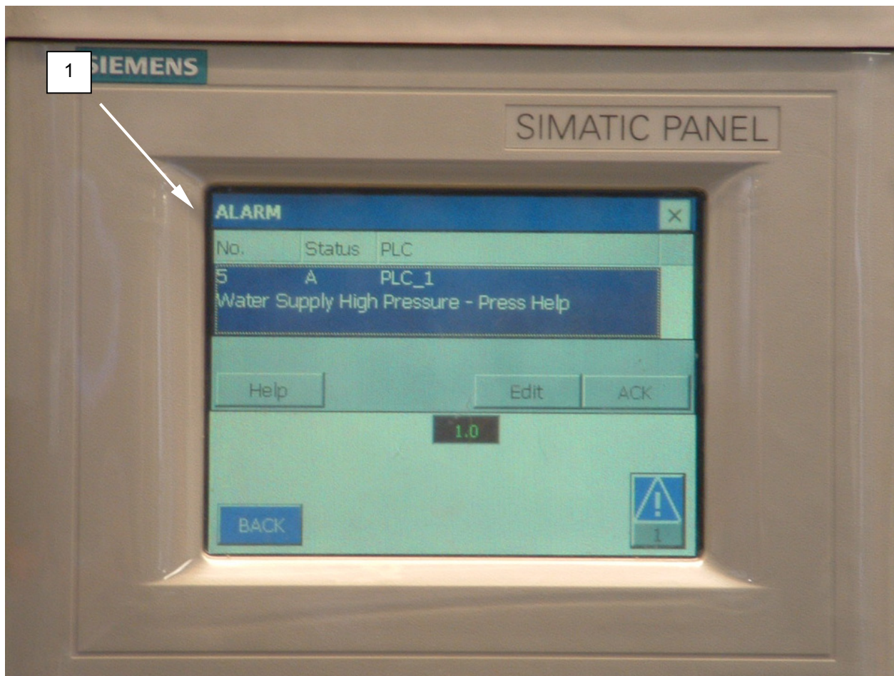
Figure 2. Water Supply High Pressure on PLC Display.
