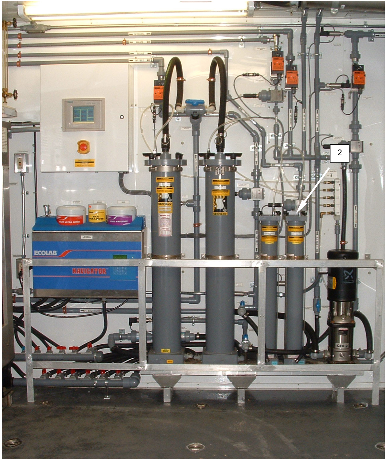
Figure 12. F-3 Carbon Filter Differential Pressure High Alarm on PLC Display.
