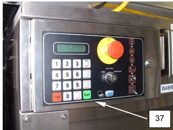
Figure 18. Purge Washer No. 2.
