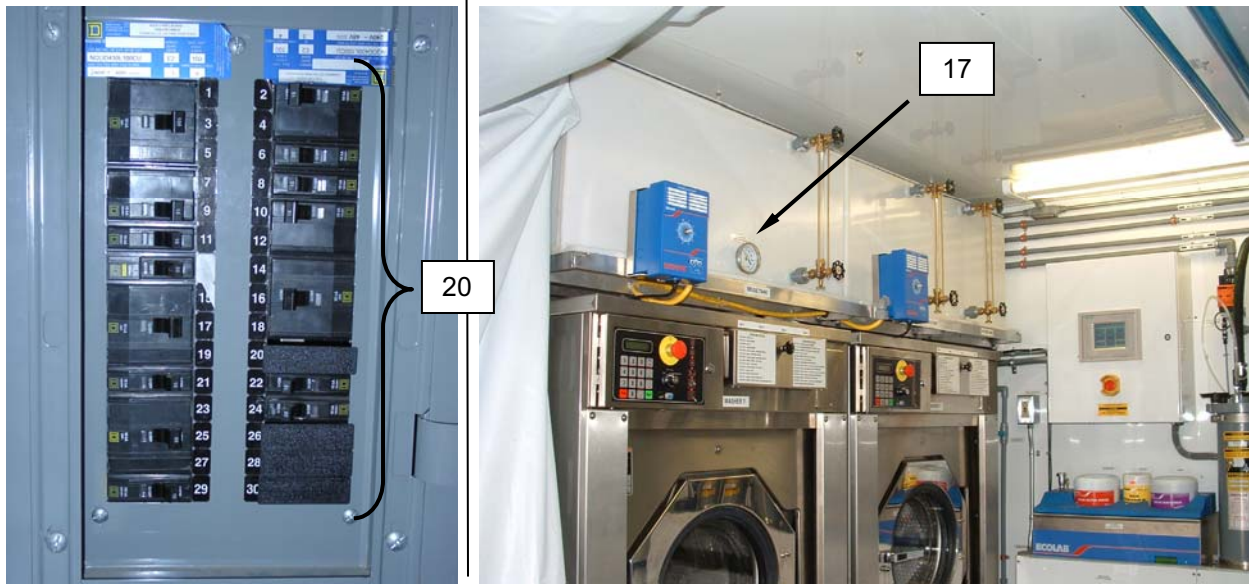
Figure 13. Switching the remaining breakers ON when temperature reaches at least 32 °F.
