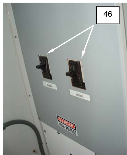
Figure 13. Check Dryer Phase Indicators.
