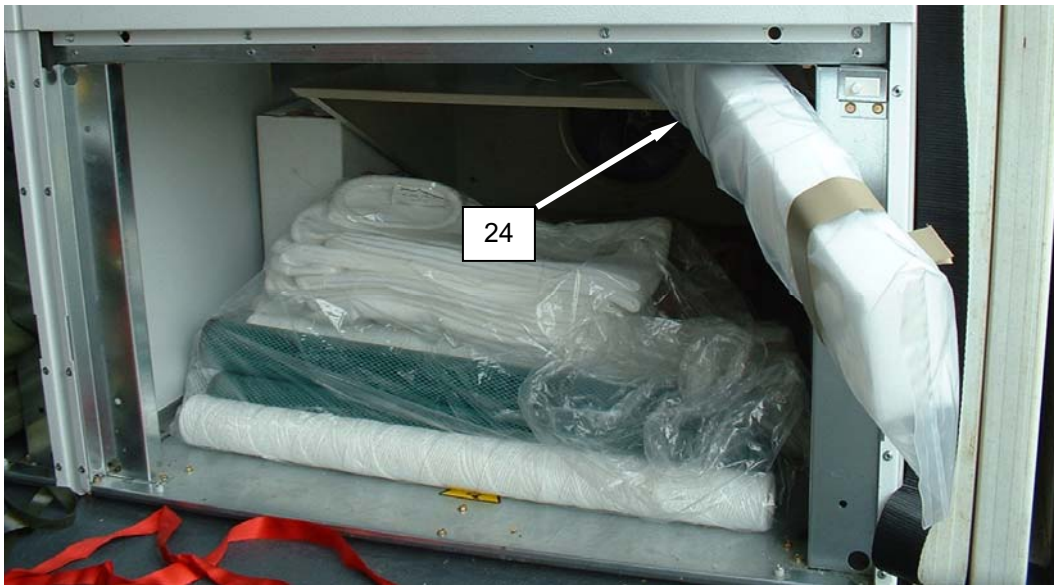
Figure 19. Water Tank Floats on Top of Lint Screen.
