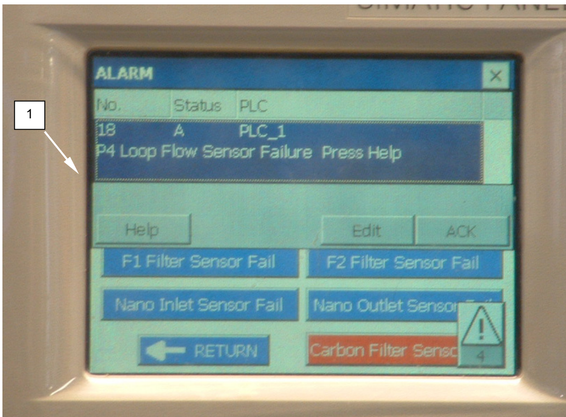
Figure 16. P4 Loop Flow Sensor Failure Alarm on PLC Display.
