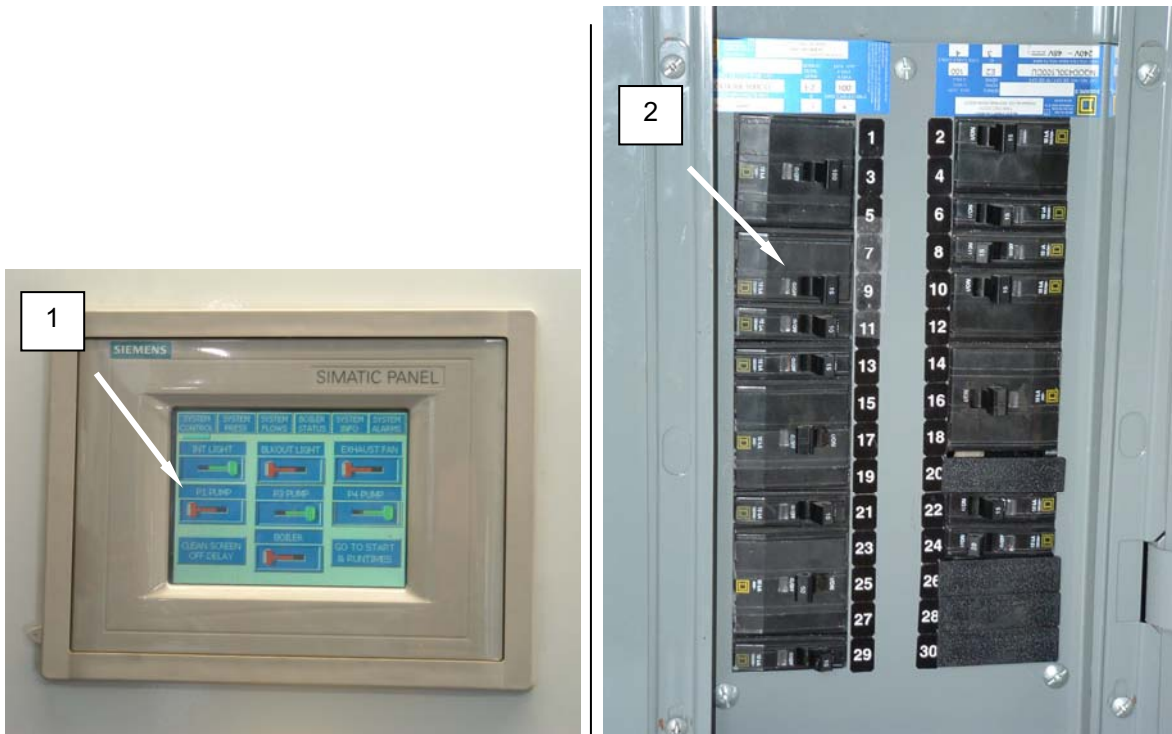
Figure 5. P-1 Pump not Operating.
