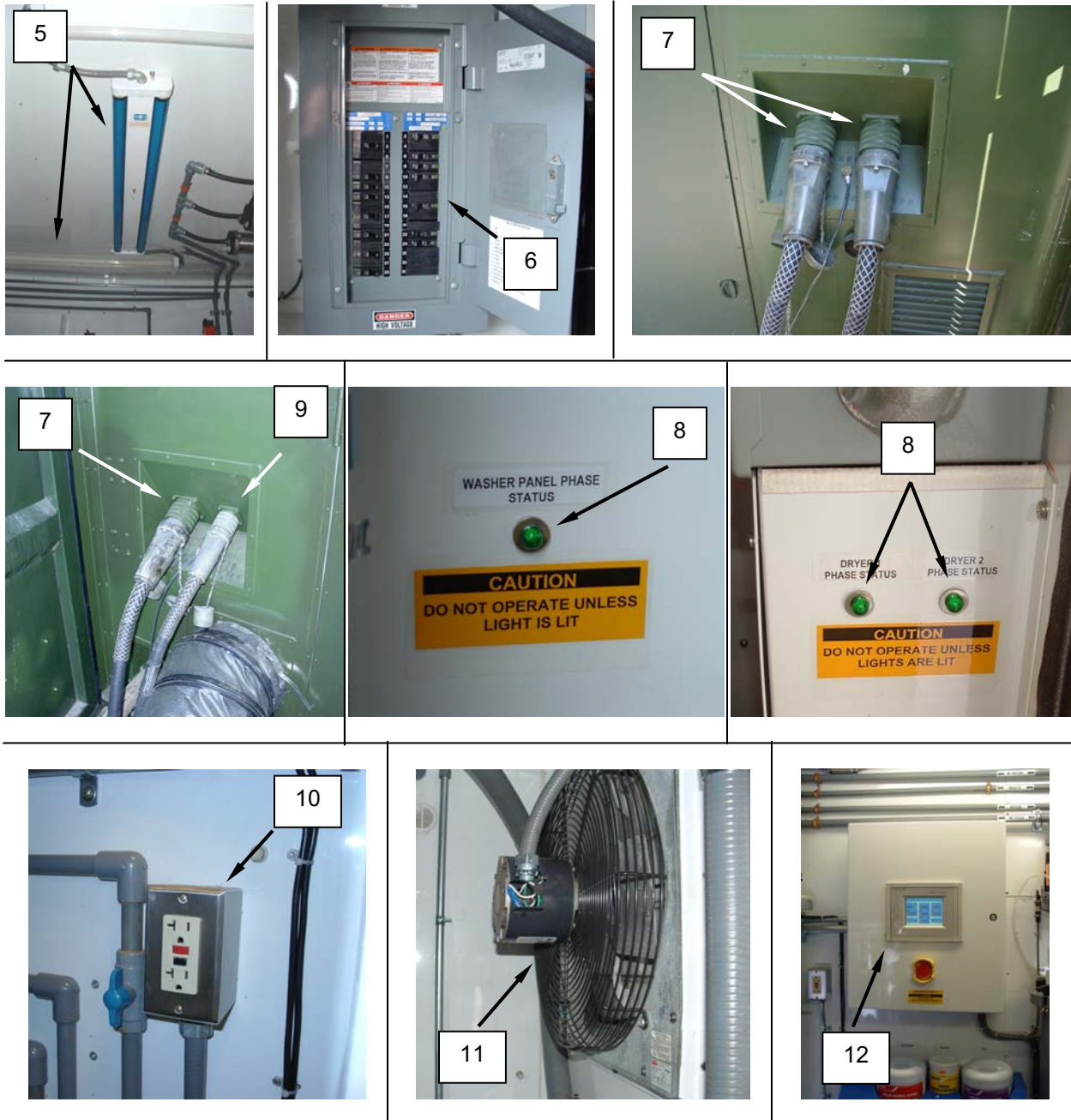
Figure 3. Lighting, Circuit Breakers, Receptacles, and Exhaust Fan.
