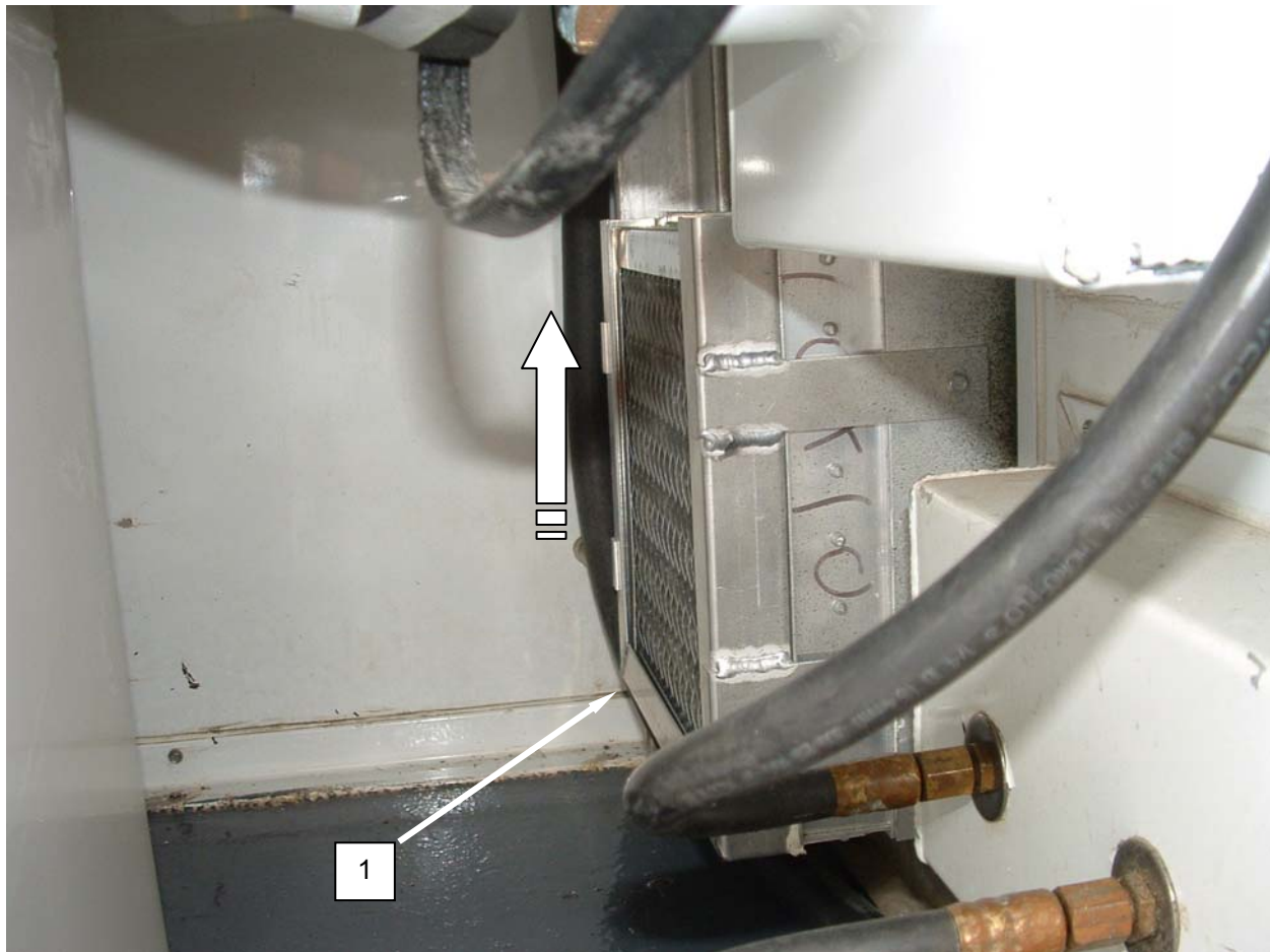
Figure 4. Replace the Boiler Air Filter.
