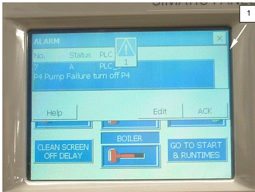
Figure 24. P4 Pump Alarm on PLC Display.
