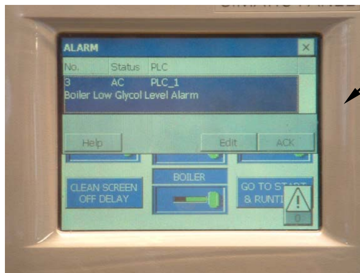
Figure 9. Boiler Low Glycol Alarm on PLC Display.
