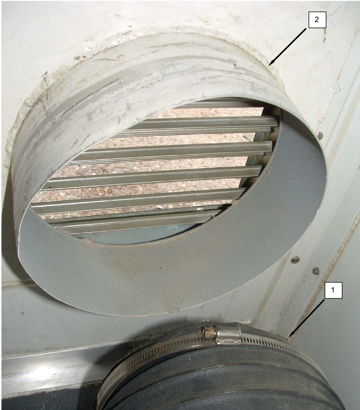
Figure 1. Dryer Exhaust Vent.
