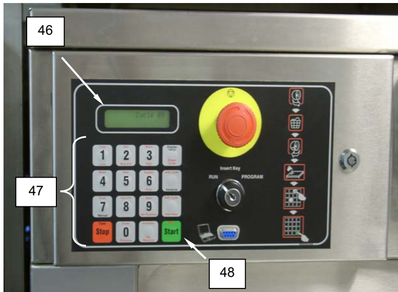
Figure 24. Washer Control Panel.
