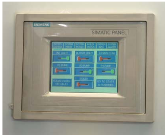
Figure 8. Boiler High Temperature Alarm on PLC Display.
