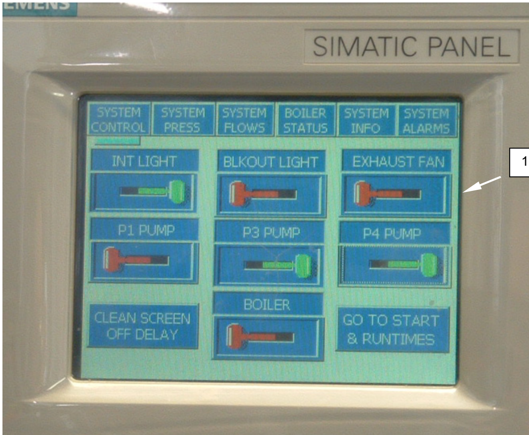
Figure 14. Reuse Loop Flow Sensor Failure Alarm on PLC Display.
