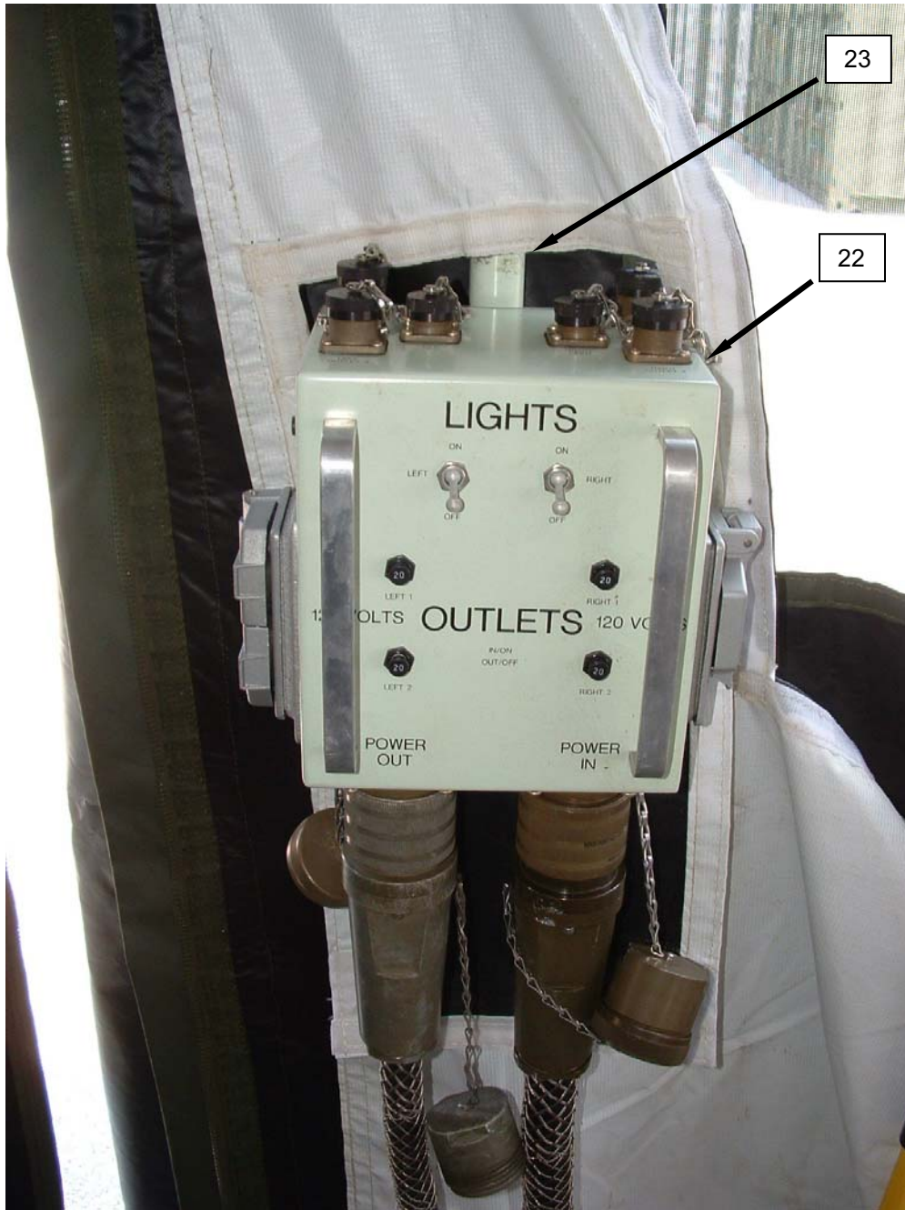
Figure 27. Remove Distribution Box and Stand during NBC Imminent or Actual Attack.
