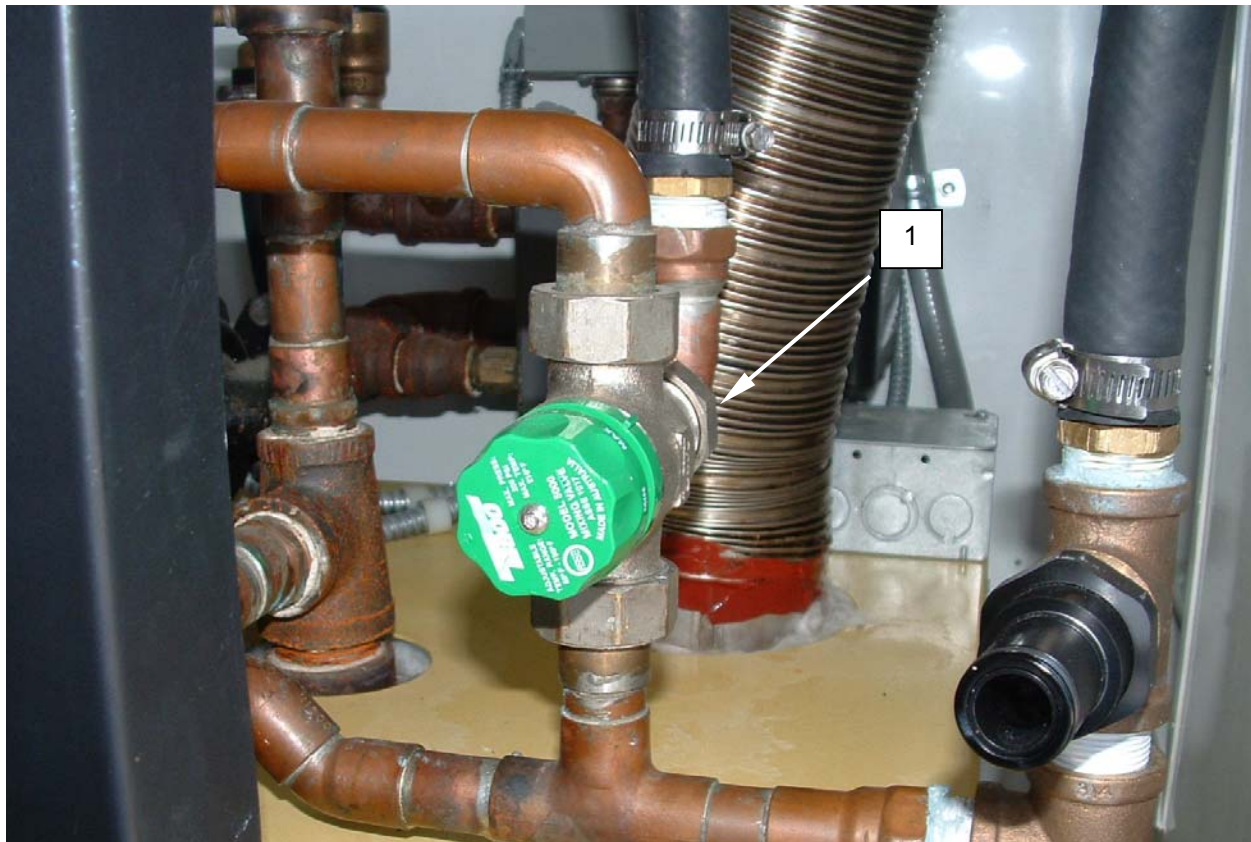
Figure 11. Boiler Operating, doesn't Heat Washer/Soap Dispenser Water.
