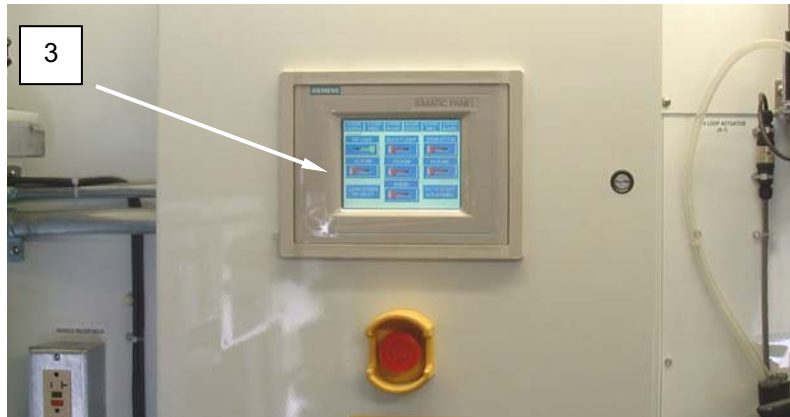
Figure 3. PLC Control Panel.
